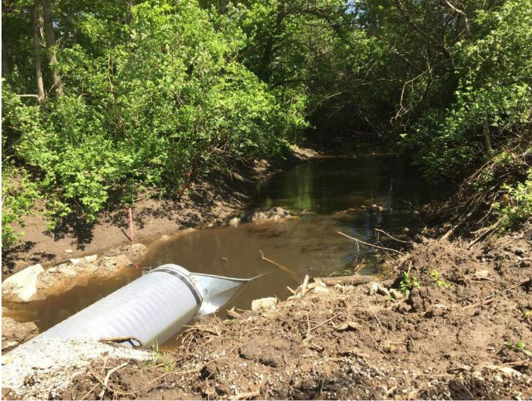
11. Stream located just east of the project area, facing south. Stream has limited flight path for use as bat foraging habitat (4-27-2017).
