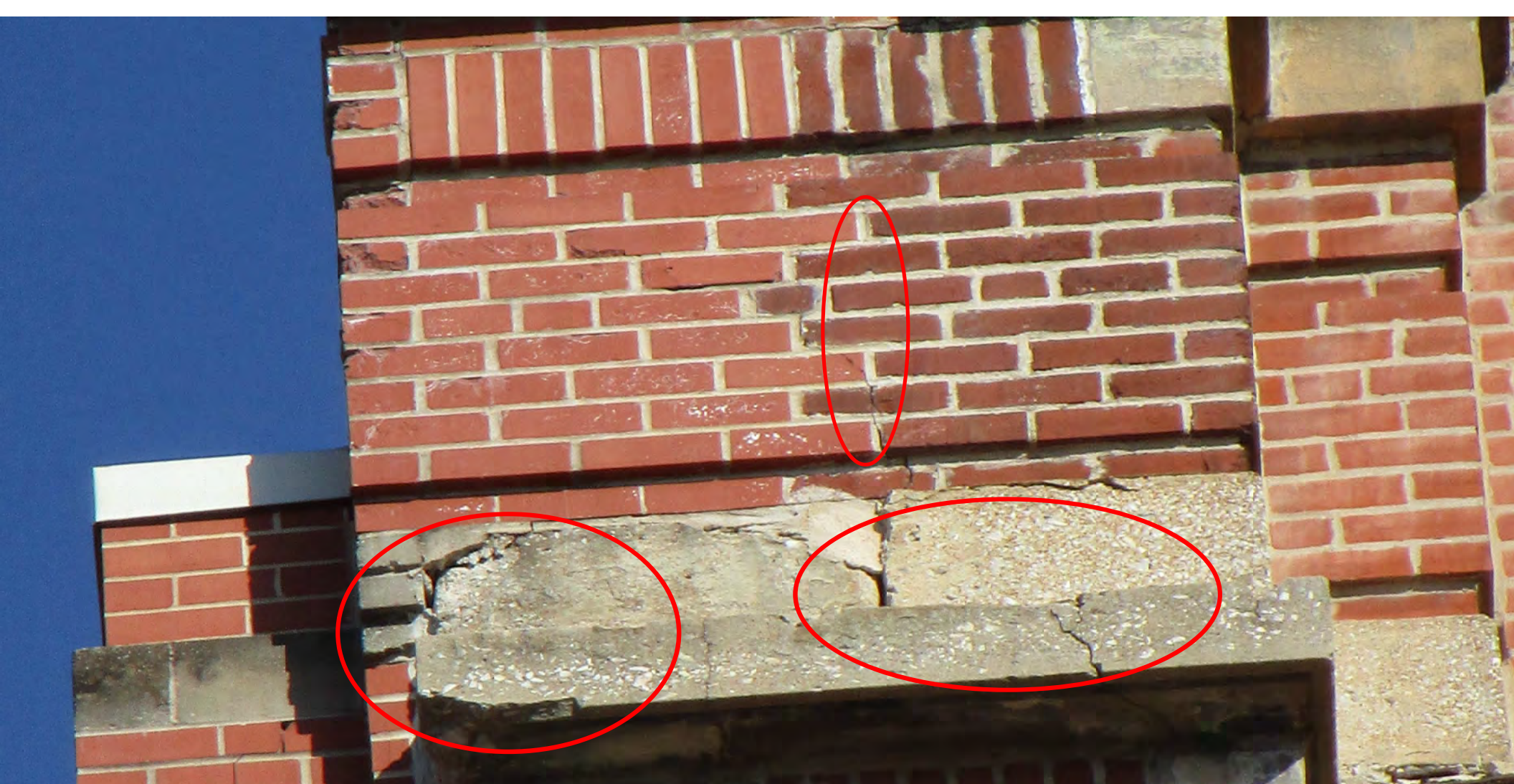
Fractured Brick & Concrete at Southwest Corner Above Sixth Floor
